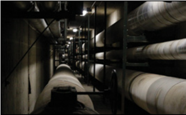
This steam tunnel houses pipes that run all over campus.
