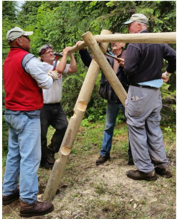
Chuck, Mike, Hank, and Carl aligning the top rail to a post frame.
